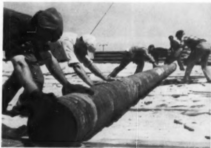
Spanish crews work on the POL line (petroleum, oil and lubricants), which will service U. S. air bases. The line starts at Rota, a Spanish Port across from Gibraltar and runs to Zaragoza in northeast Spain
